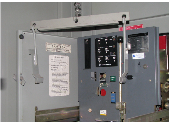
Photo 3a. This circuit breaker is ready to be lifted from its extension arms.
