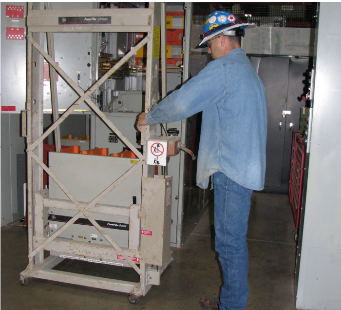
Photo 4b. This technician is using the lifting platform to install a medium-voltage draw-out type vacuum circuit breaker.
