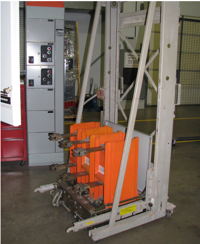
Photo 4a. Here's an example of a vacuum circuit breaker lifting platform.
