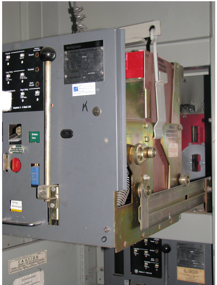
Photo 3b. This circuit breaker is ready to be lifted from its extension arms.
