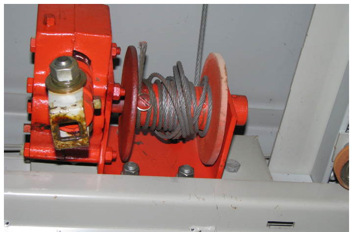
Photo 2. This is a typical winch arrangement found on an LVPCB line-up.
