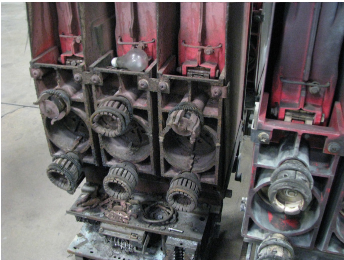
Photo 8. Note the results of serious maintenance neglect.
